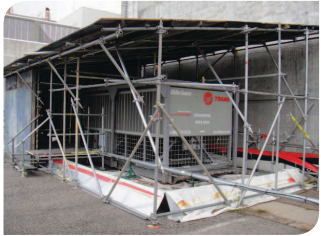
The rental equipment had to fit seamlessly with the existing cooling system piping.
