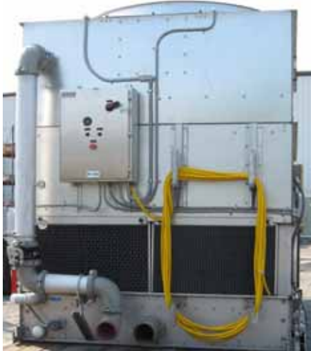
Figure 1. 250 ton CT Piping and Control Panel
