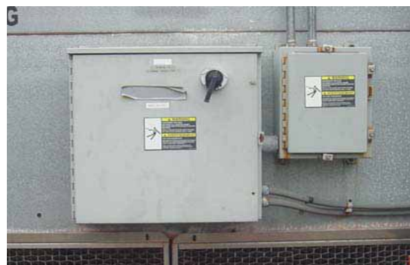
Figure 4. Circuit Breaker - All other 500 ton Towers
