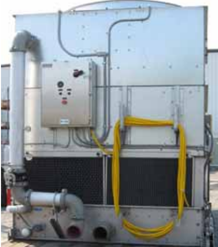
Figure 5. 250 ton CT piping and control Panel
