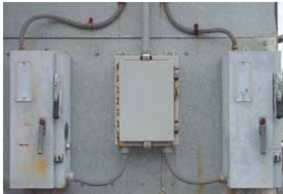
Figure 3. Fused Disconnect CSCT05000F0AC
