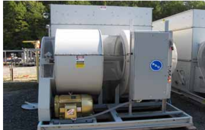
Figure 2. 270 ton CT Motor Control Panel
