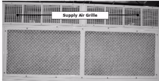
Figure 10. Supply Air Grille
