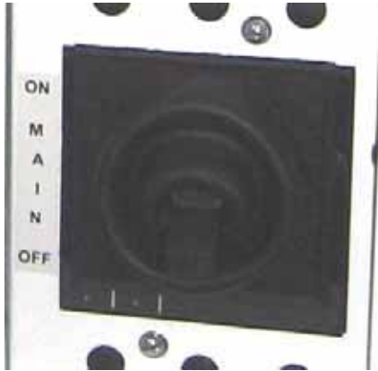
Figure 12. Main Unit Circuit Breaker
